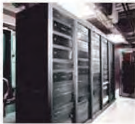
Gangable Floor-standing Enclosures
